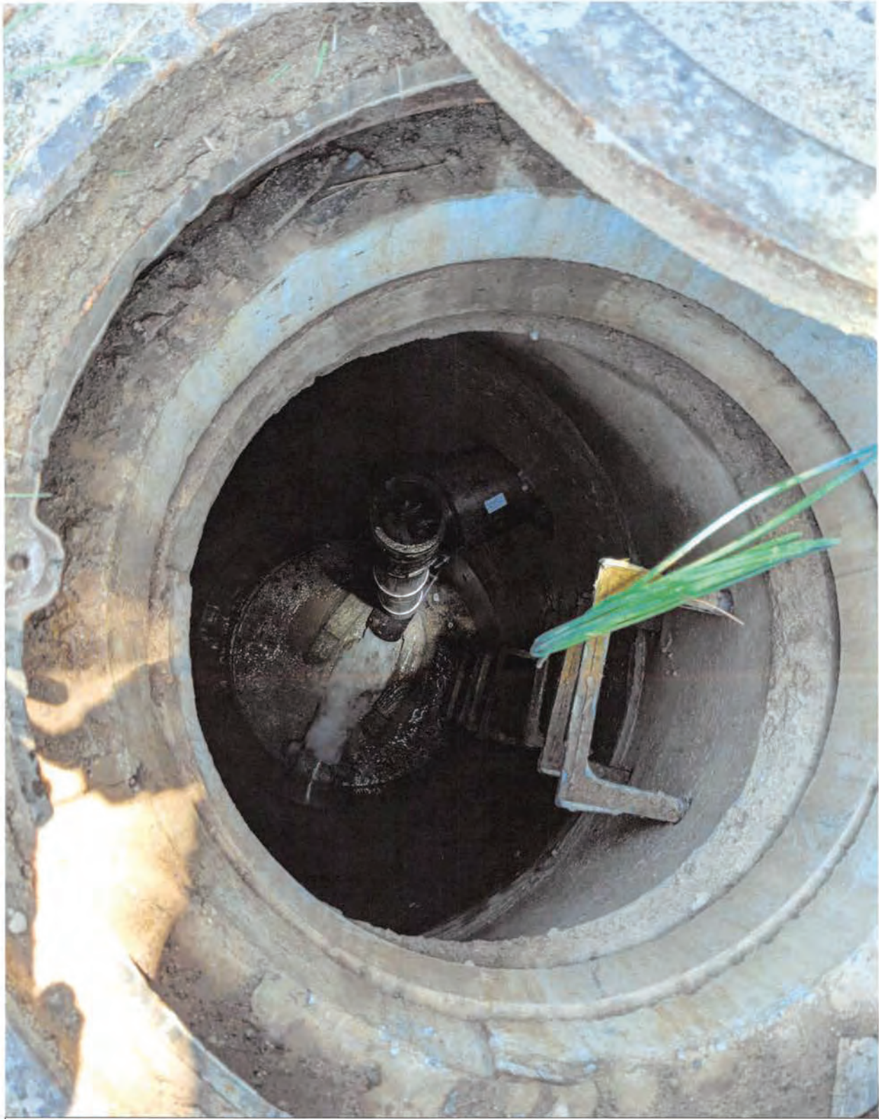
Water from Lake Edgewood Test Flowing into Genoa- Oceola Gravity Sewer
