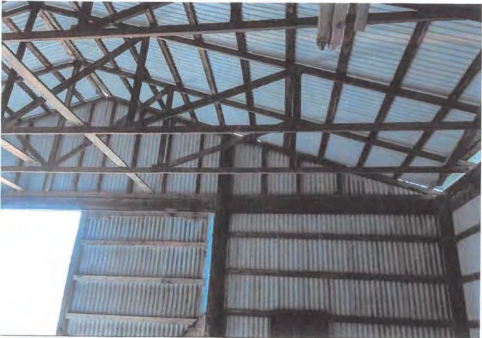
Picture 8 – Openings Between Roof and Fascia Boards on Larger Building
