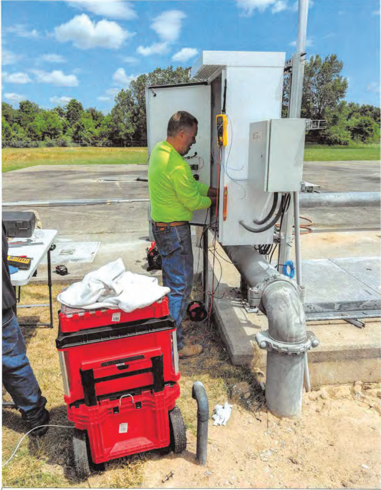
Wiring of New Pump Control and Instrumentation Panel Installed On- Site of Lake Edgewood SST
