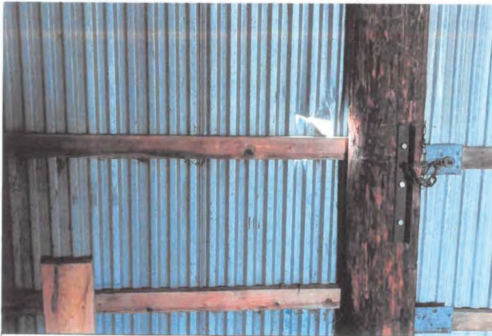
Picture 6 – Holes in Sheeting on Larger Building
