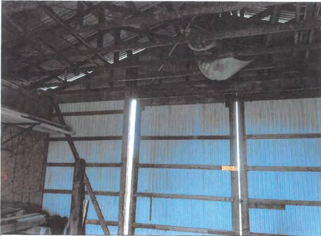
Picture 12 – Rear of Smaller Pole Building Showing Large Gaps Between Walls and Roof
