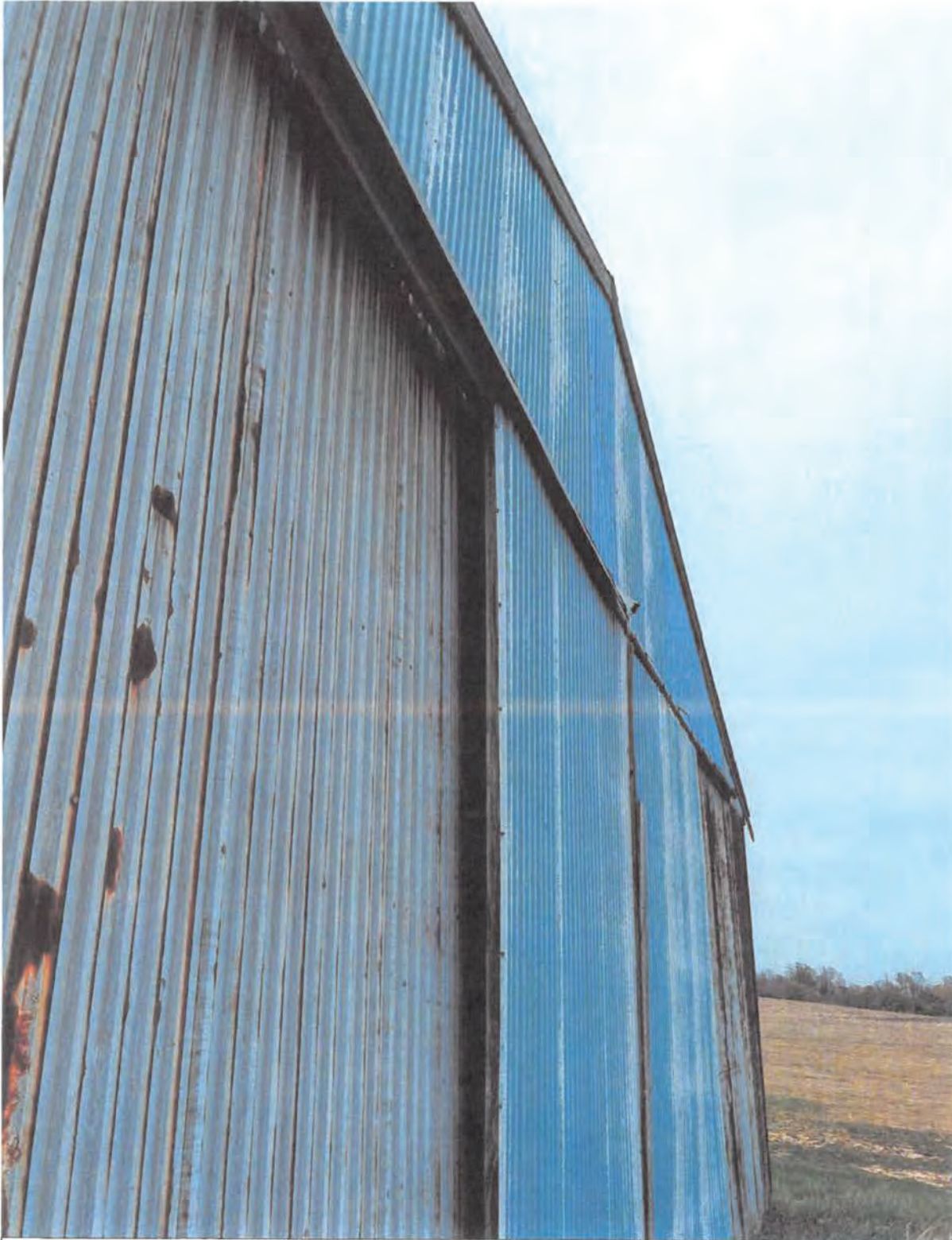
Picture 9 – Large Gaps Between Sliding Doors and Walls on Rear of Larger Pole Building
