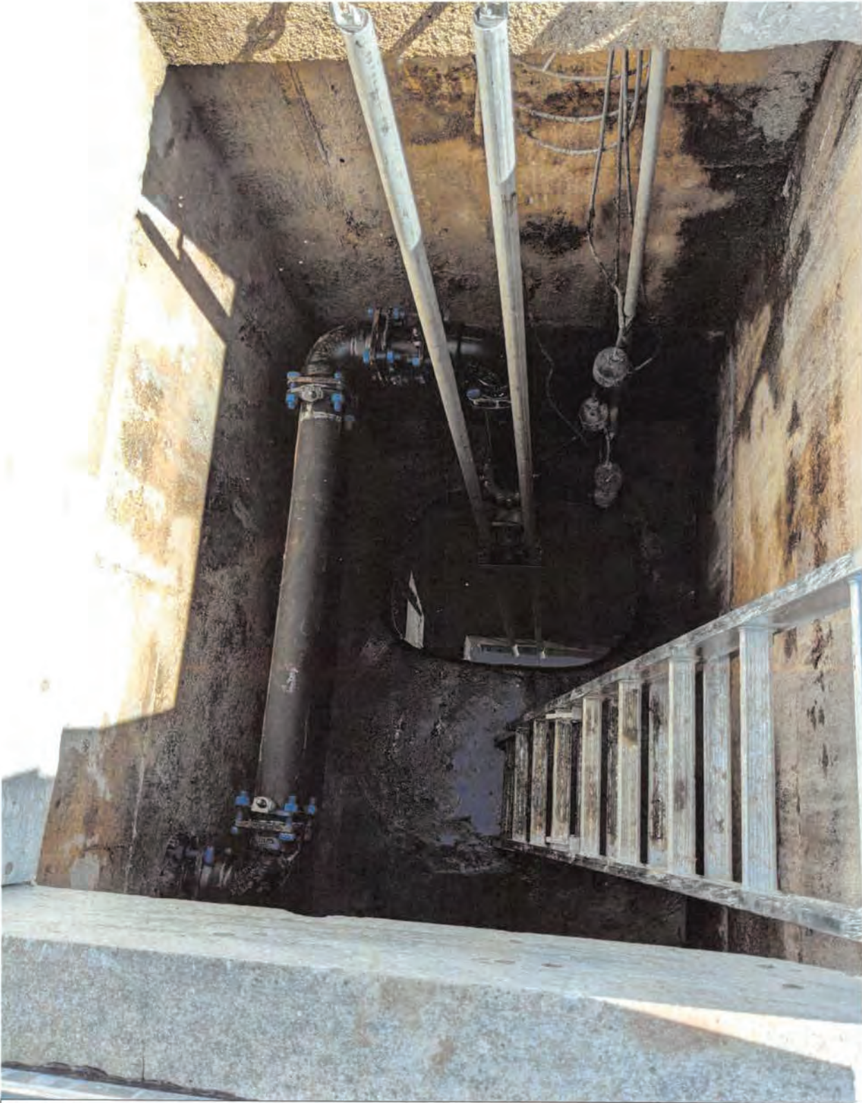
New piping rails installed in existing decant chamber to become pump chamber to Genoa-Oceola
