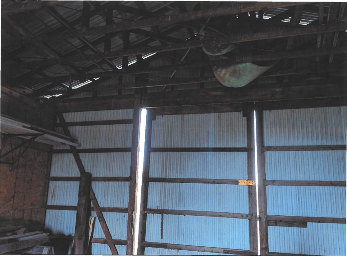
Picture 12 – Rear of Smaller Pole Building Showing Large Gaps Between Walls and Roof
