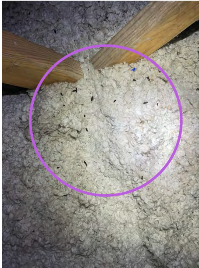
Bat droppings in the attic space.
