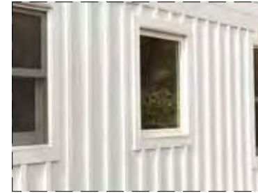
M-1: Exterior Siding Manuf: James Hardie Type: Board and Batten Vertical Siding Color/Finish: Arctic White
