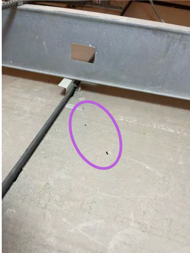
Mouse droppings above the drop ceiling.
