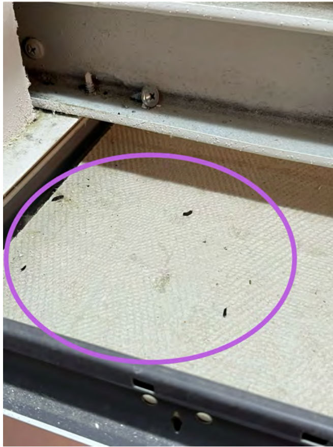
Mouse droppings above the drop ceiling.
