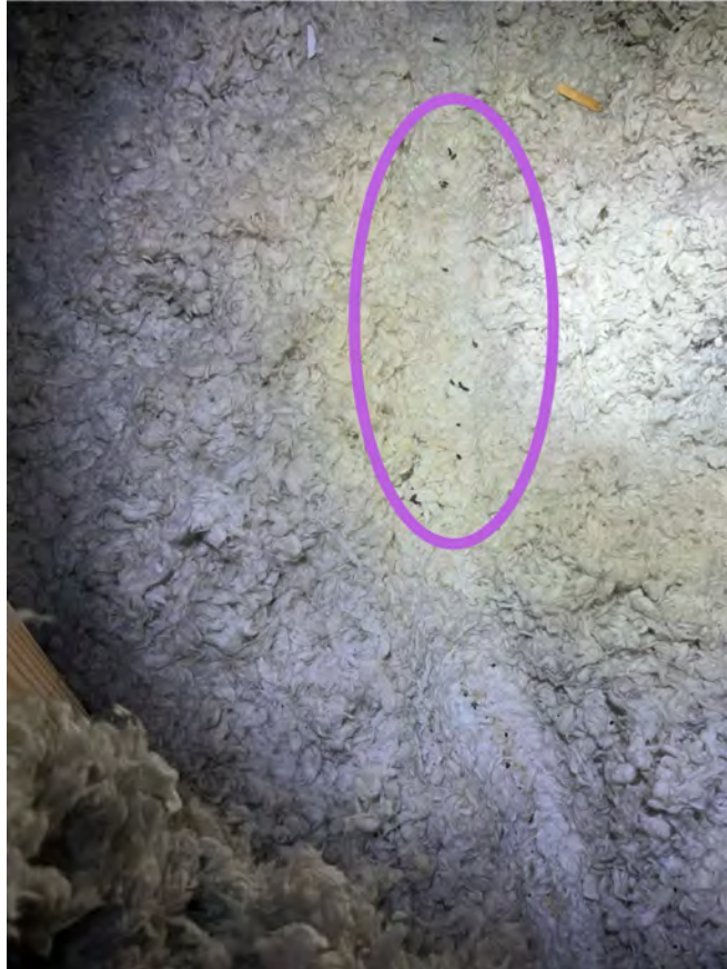
Mouse droppings in the attic space.
