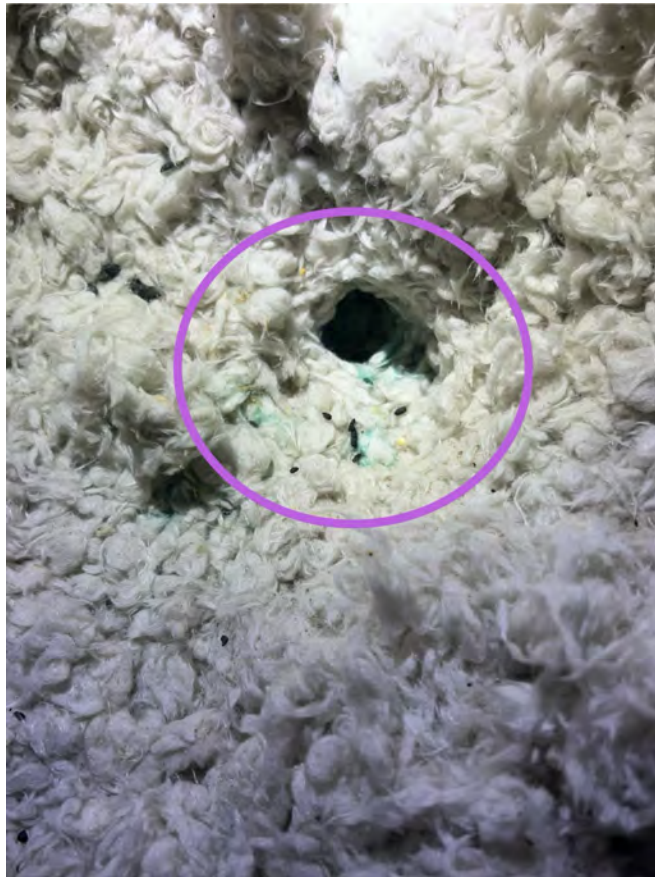
Mouse tunnel and mouse droppings in the attic space.
