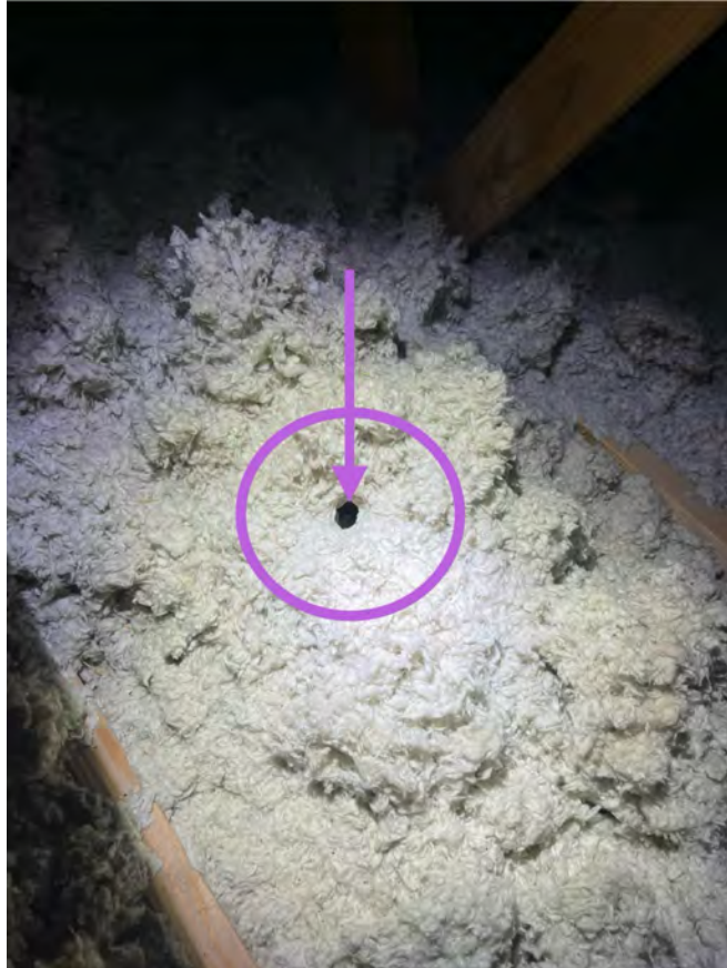
Mouse tunnel through the attic insulation.
