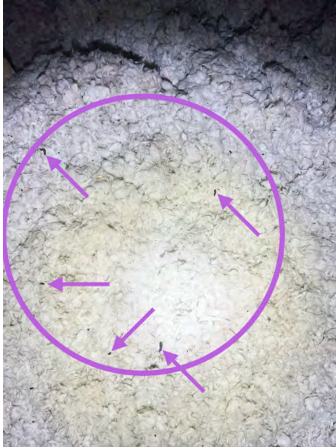
Bat droppings throughout the attic space.
