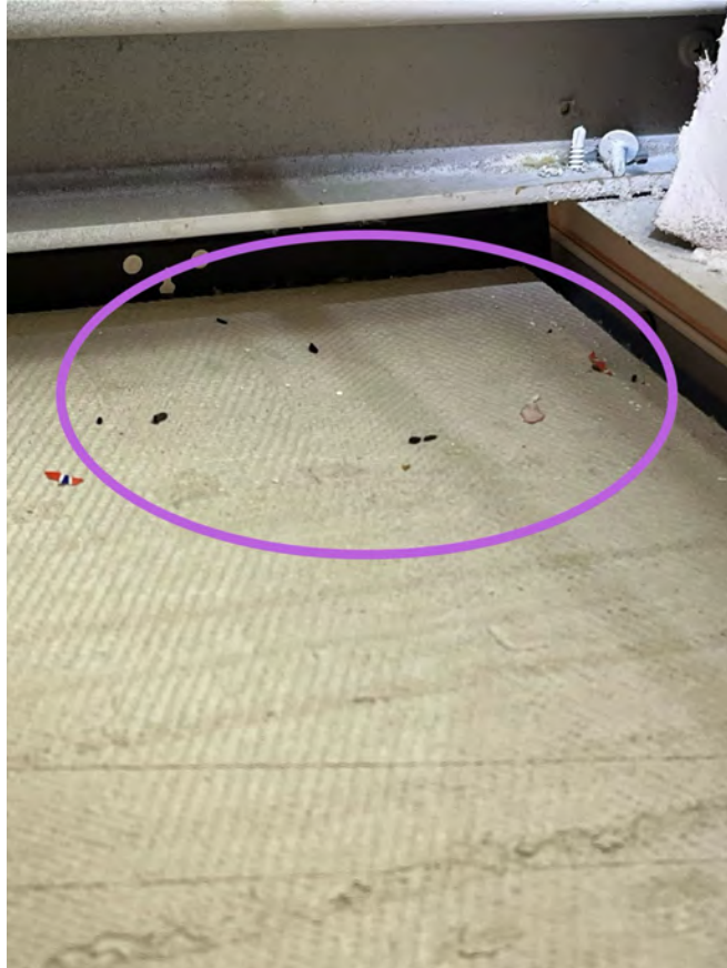
Mouse droppings above the drop ceiling.
