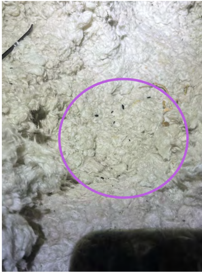
Mouse droppings in the attic space.
