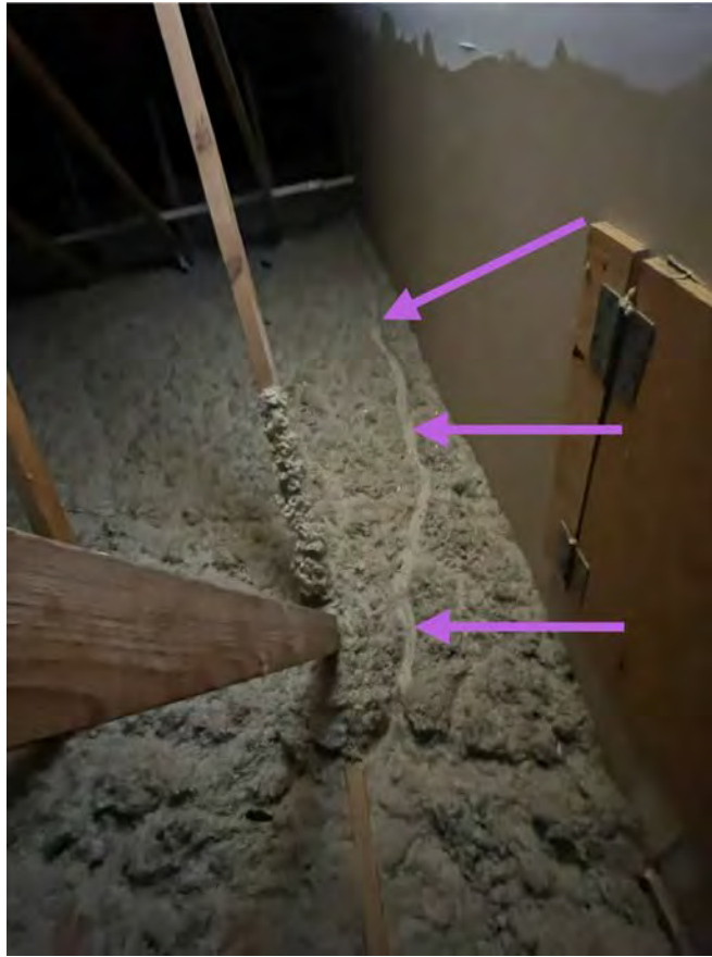
Mouse pathway through the attic insulation.
