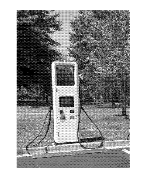
F EV charging station TOTAL OF 4-CONDITIONS
