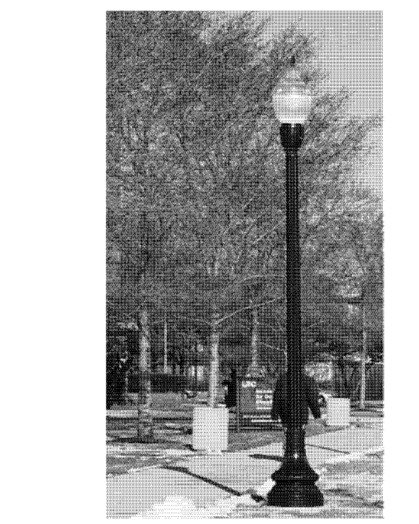
A decorative pole and light (5-CONDITION) DECORATIVE BLVD. ISLAND SITE FIXTURE LIGHTS AND ALUMINUM POLE.
