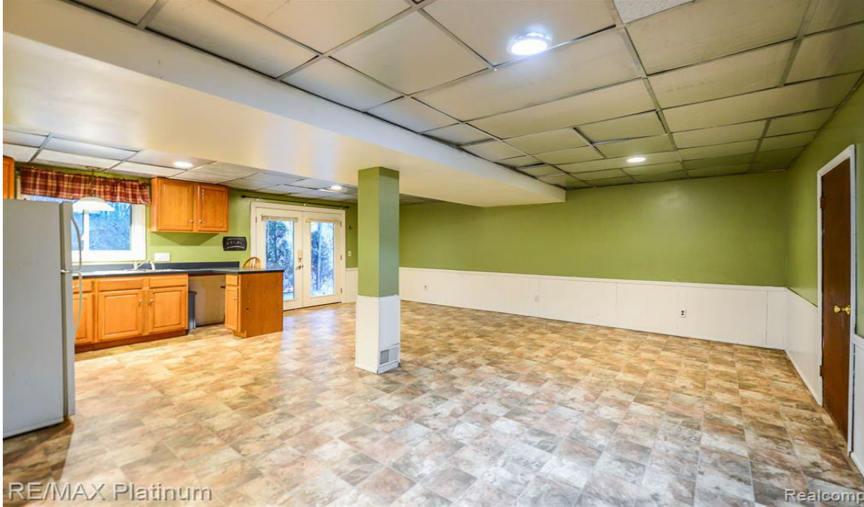
Figure 4 Picture of existing basement living room area with walk-out basement door. This area will be updated.
