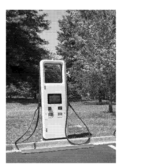
F EV charging station TOTAL OF 4-CONDITIONS
