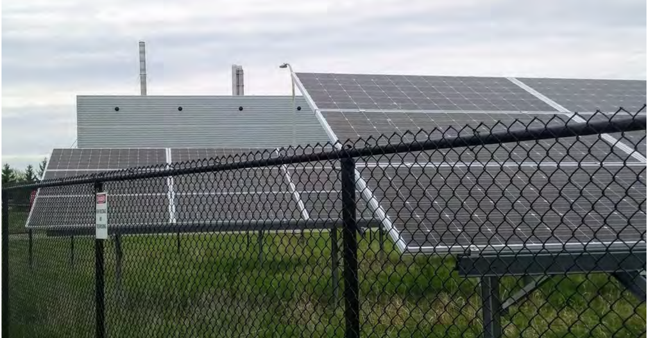
Consumers Energy - Western Michigan University, Business Technology and Research Park solar garden. Photo by Mary Reilly.
