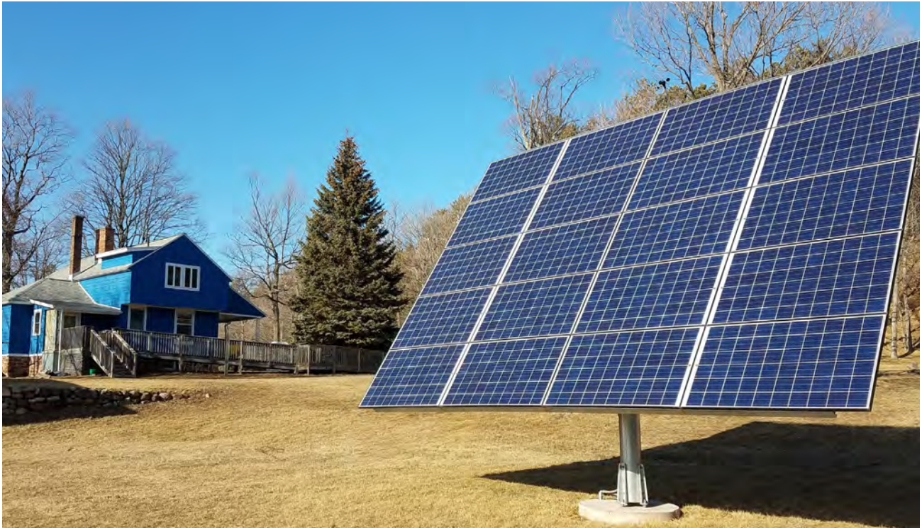
Ground-mounted monopole SES. Photo by Bradley Neumann.
