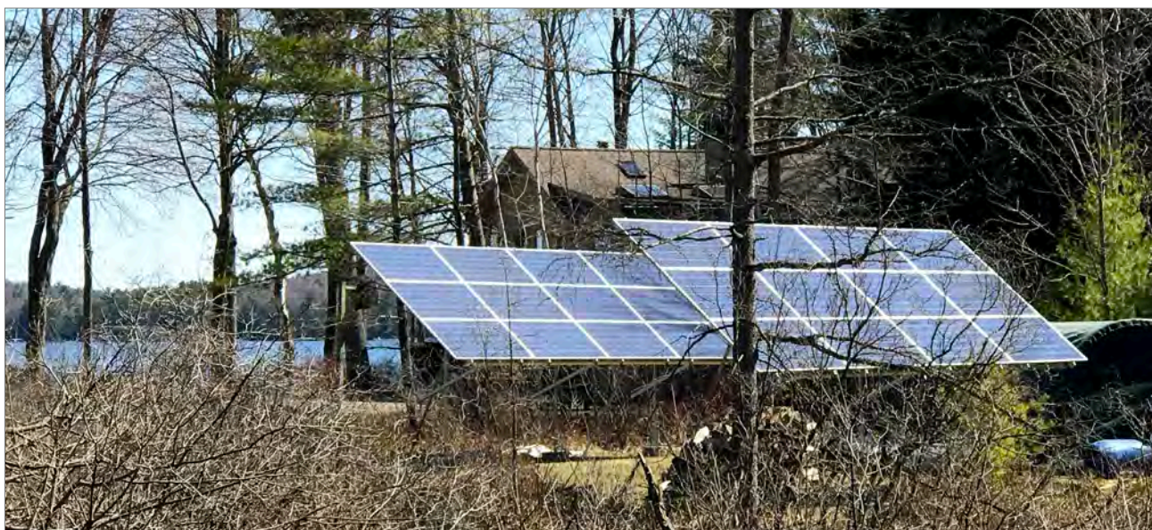
Ground-mounted SES, Grand Traverse waterfront. Photo by Mary Reilly.
