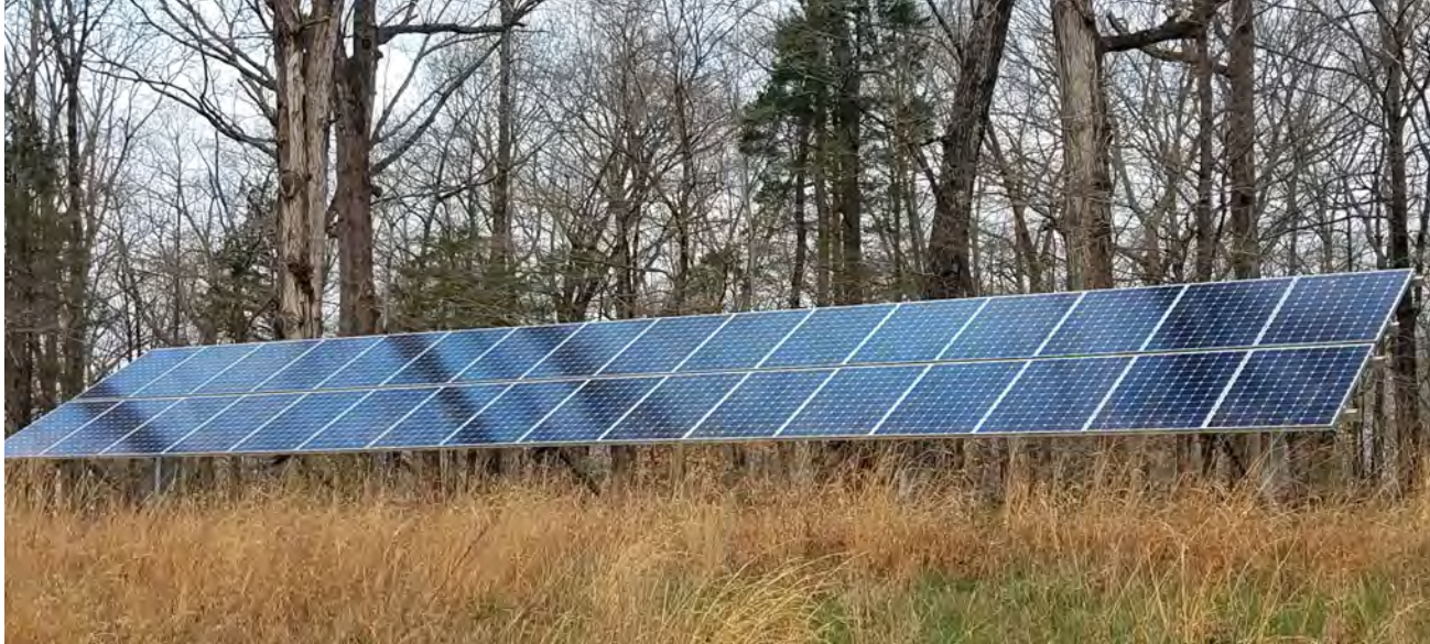
Ground-mounted SES in rural setting. Photo by Bradley Neumann.
