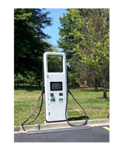
F EV charging station TOTAL OF 4-CONDITIONS
