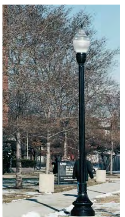
A decorative pole and light (5-CONDITION) DECORATIVE BLVD. ISLAND SITE FIXTURE LIGHTS AND ALUMINUM POLE.
