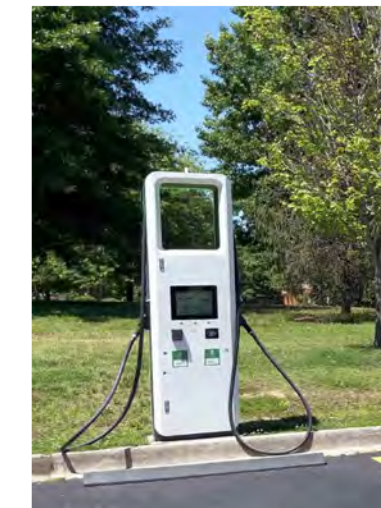
L EV charging station TOTAL OF 4-CONDITIONS
