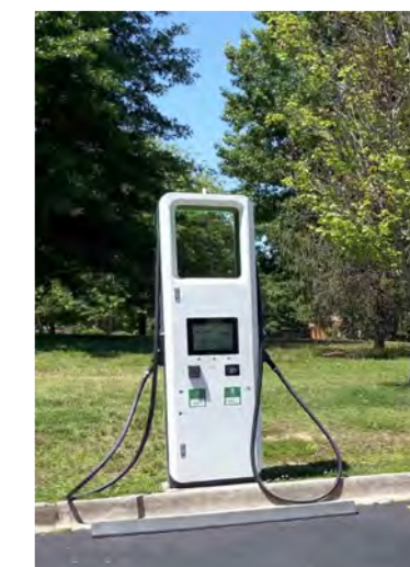
L EV charging station TOTAL OF 4-CONDITIONS
