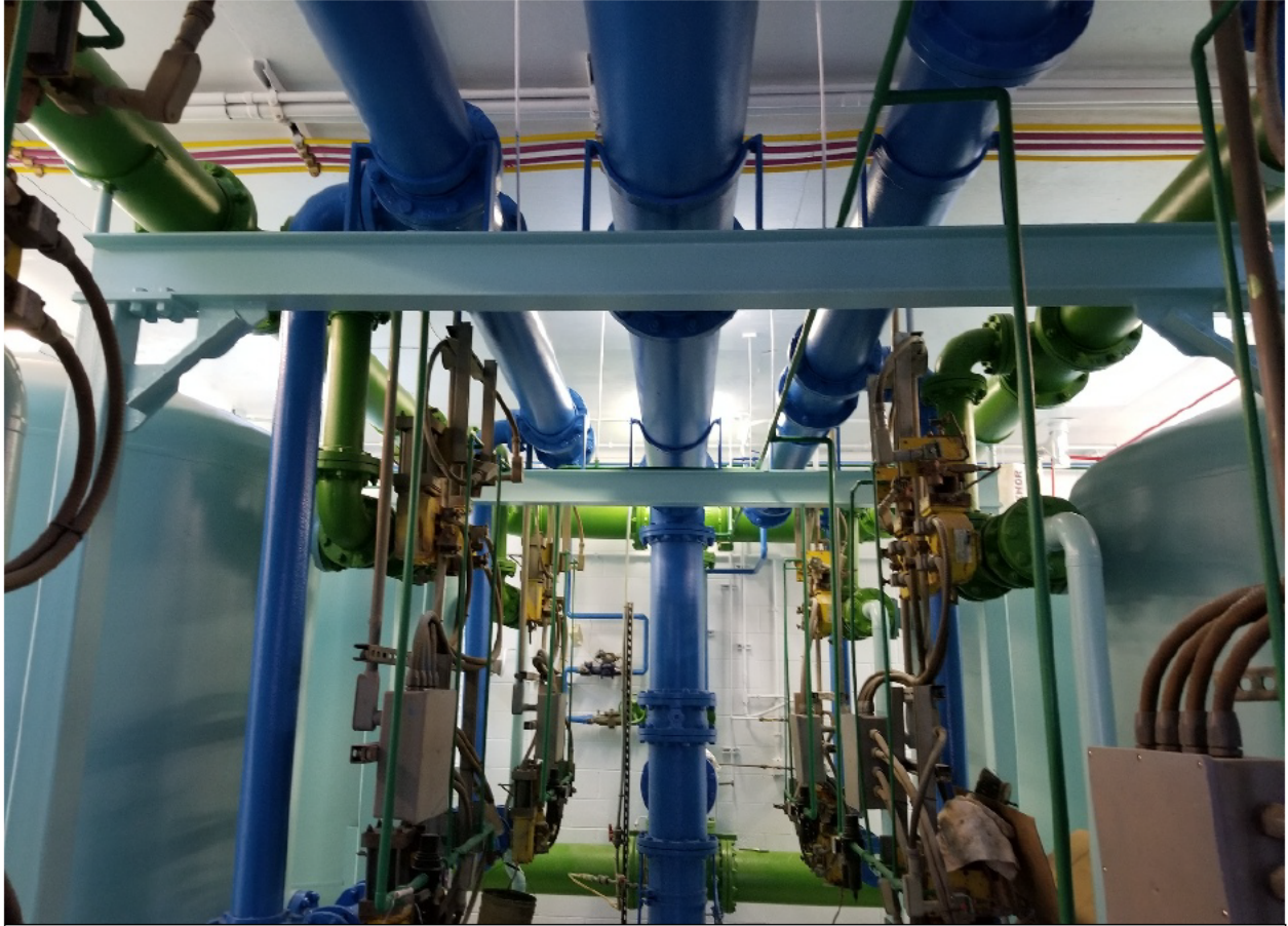
Iron Removal Filter Pipe Gallery
