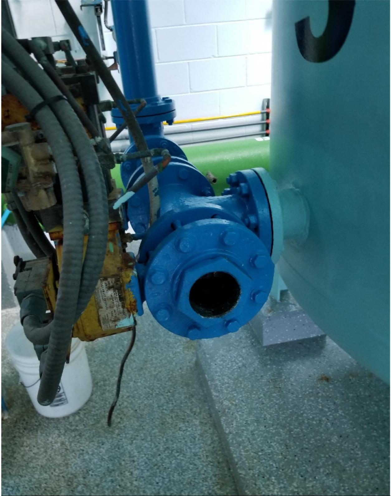
Rinse Outlet with Broken Pipe Nipple Removed
