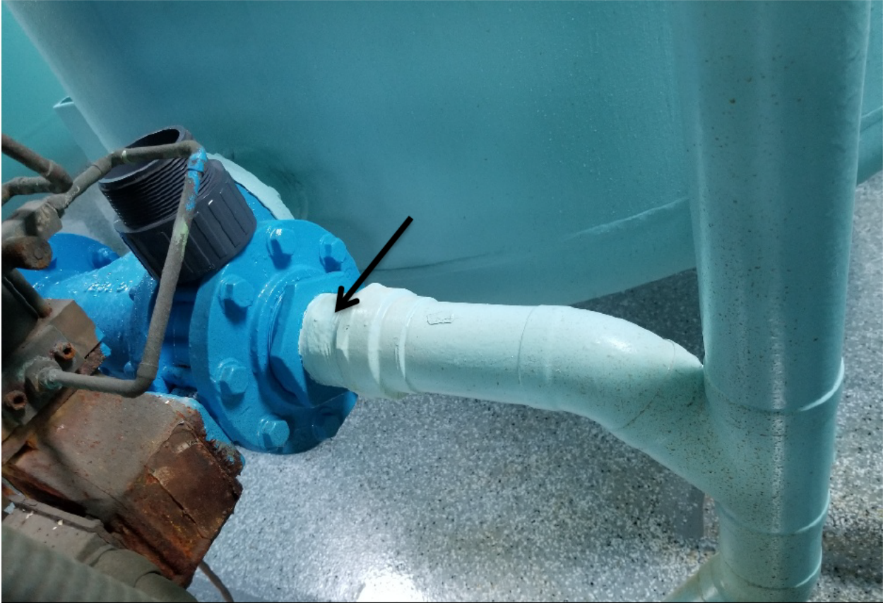
Rinse Outlet with Pipe Showing Thinning Walls
