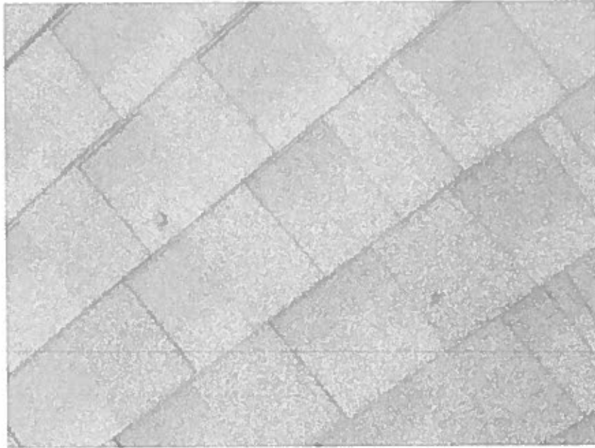
Backed out nail where leak is directly present in fire bay.
