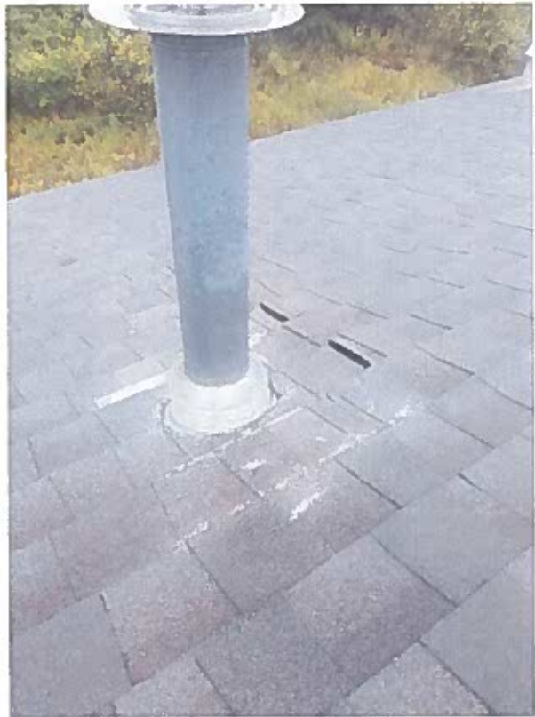
Severe buckling on north side of roof.
