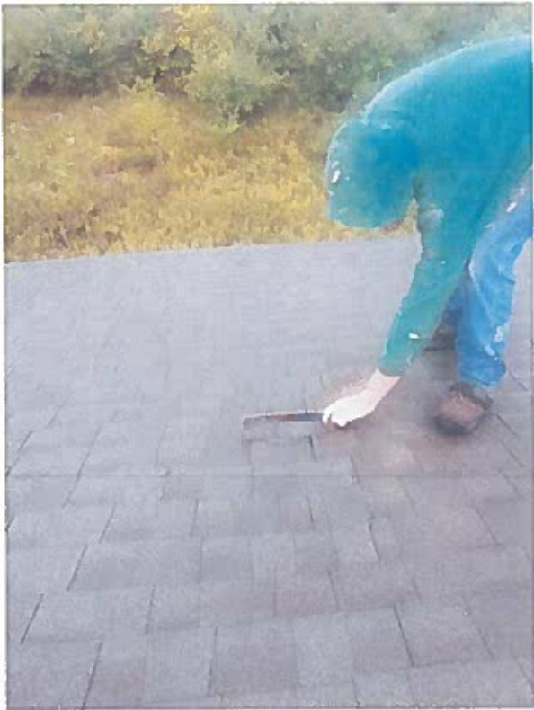
Rotted plywood where racked/stacked seams are extremely close.
