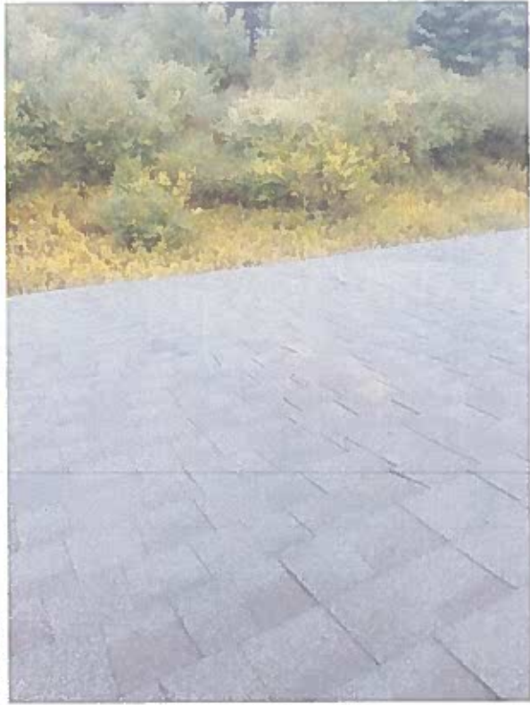
Additional rotted plywood on north side of roof.
