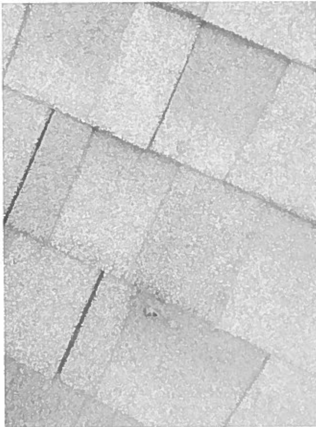
Numerous backed-out nails—a result of poor ventilation issues.
