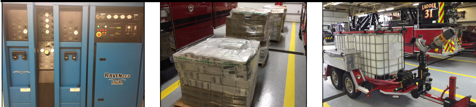
Cascade Air Filling Station, Smoke Alarms and CO Alarms, and Specialized Foam Trailer
