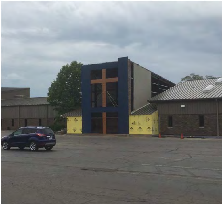
Photo 4 non matching building materials and change to site plan façade.
