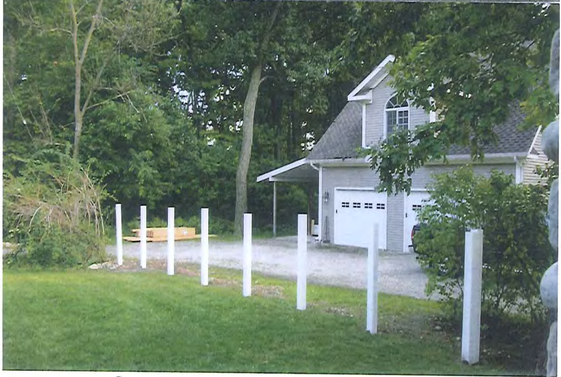
Fence posts installed completely on the property at 6483 Forest Beach Dr. before surveying done by 6471 Forest Beach property owner. Posts have been taken down and survey stakes/work done. Concrete footing material currently still below grade on property of 6483 forest Beach.
