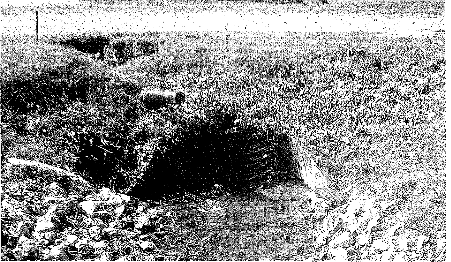
Lake Chemund Dam driveway failure due to culvert deterioration.
