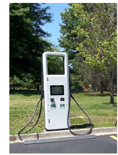
L EV charging station TOTAL OF 4-CONDITIONS
