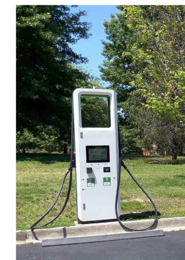
L EV charging station TOTAL OF 4-CONDITIONS
